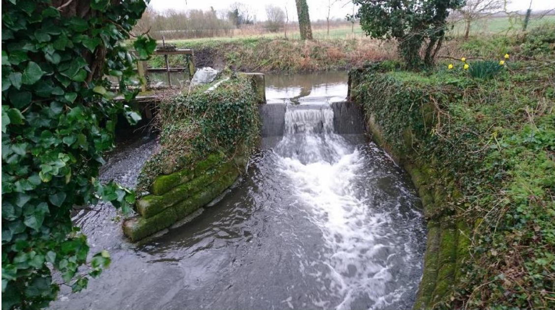
Before: Weir bypass channel which was impassable to fish during most flow conditions.
